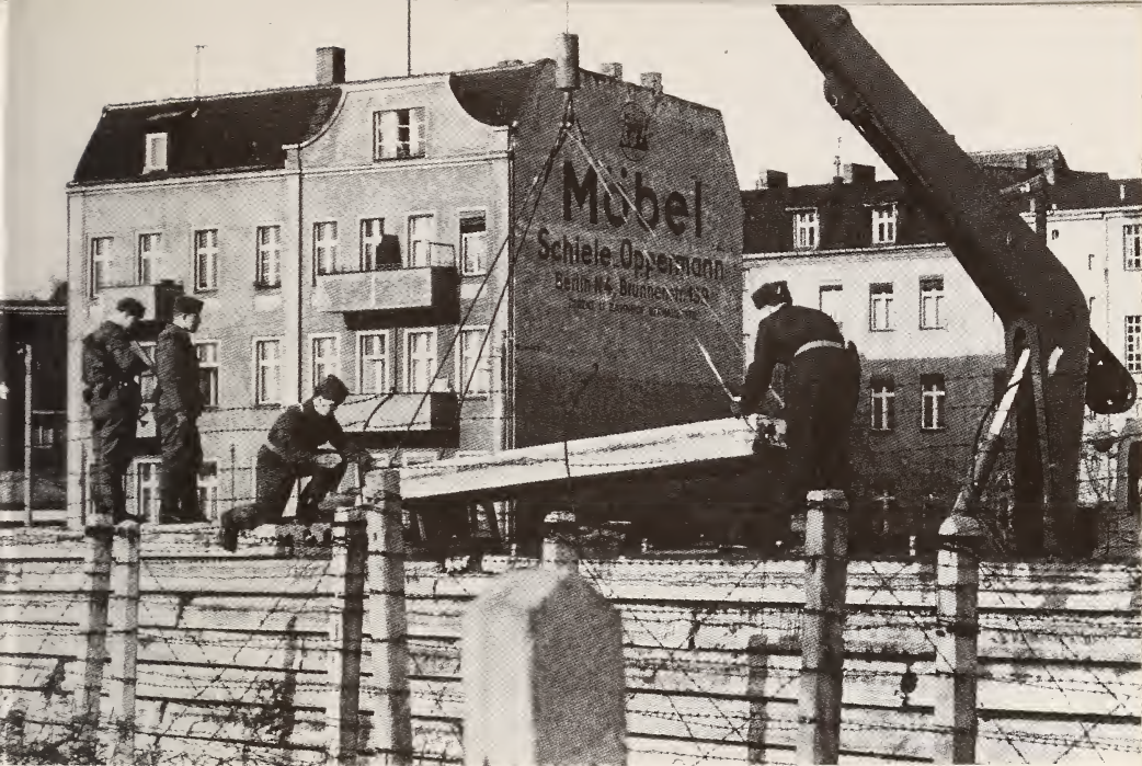
Members of the People's Police reinforce the Berlin Wall with concrete slabs in 1965. Courtesy United Press International
